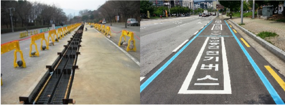
Figure 1.4: Charging points for WPT. On the left there is a charging point in construction and on the right one already working (from [9] and [10]).
